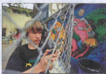
Old wire from a chain link fence is removed by Myles Adams.
